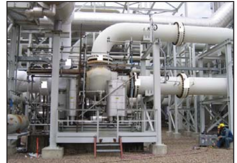
Figure 2: Expander interface data have to be collected to design replacement equipment
